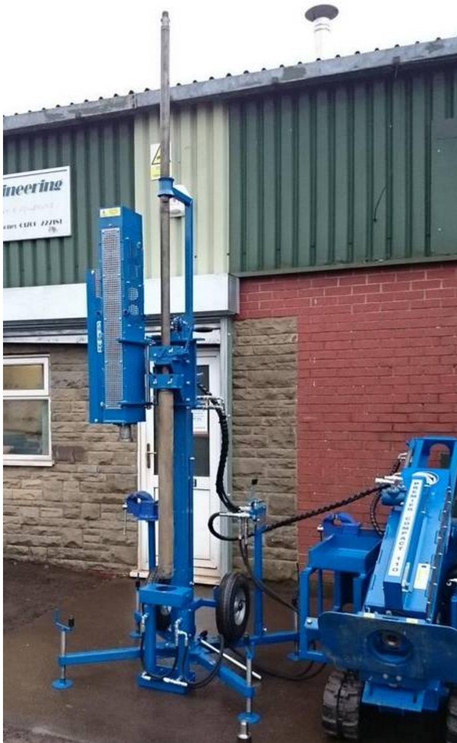
Figure 2 Mod rig in extraction setup showing the upper rod guide system were the jacks have first been used to extract the drill string then the mast pullback has been used to extract both rods and sampler clear above the jack thus allowing the jack and sampler to be removed and the next sampler fitted and lowered into position, unique to the rig.
